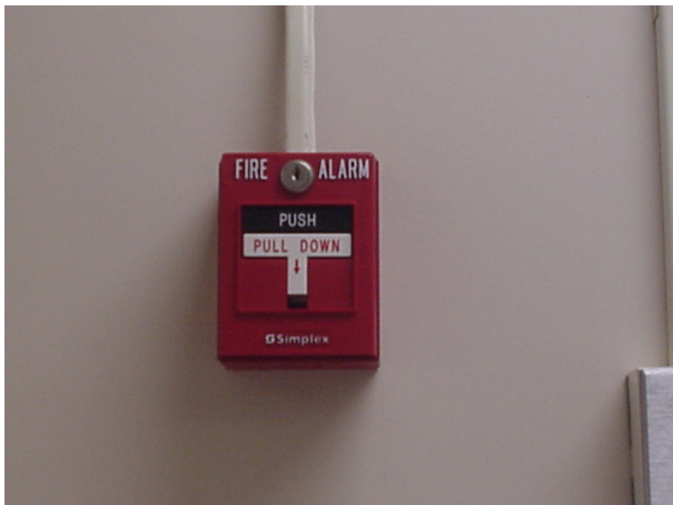
Fire Pull Station
