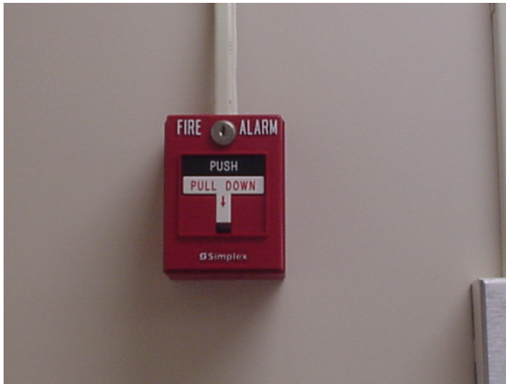
Fire Pull Station
